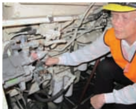
Peter Yee inspects a Unicla compressor, still working efficiently under layers of fine coal dust in a coal excavator
